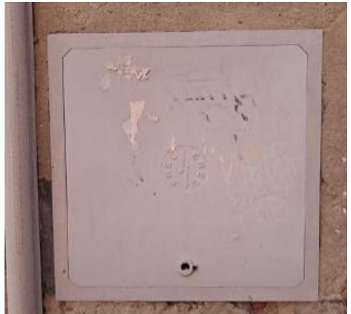
(Example of minimally altered ENEL box)
